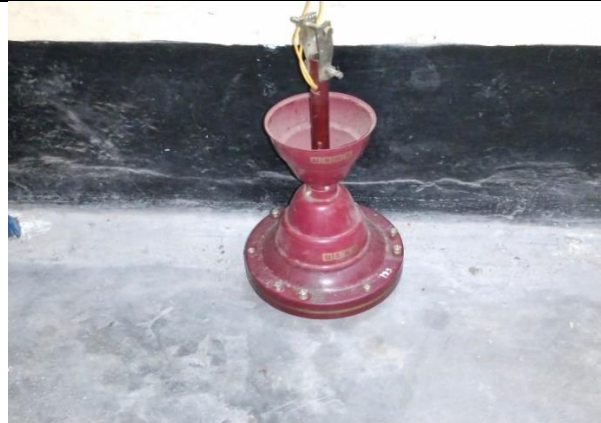
Performing routine maintenance on electrical fans. The accumulation of dust and debris can hinder the fan's performance. Regular cleaning of the grilles, blades, and motor housing is necessary to maintain optimal operation, ensure smooth airflow & save energy.
