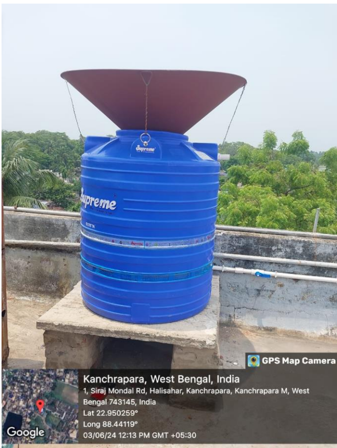
RAIN WATER HARVESTING RESERVOIR ON ROOFTOOP
