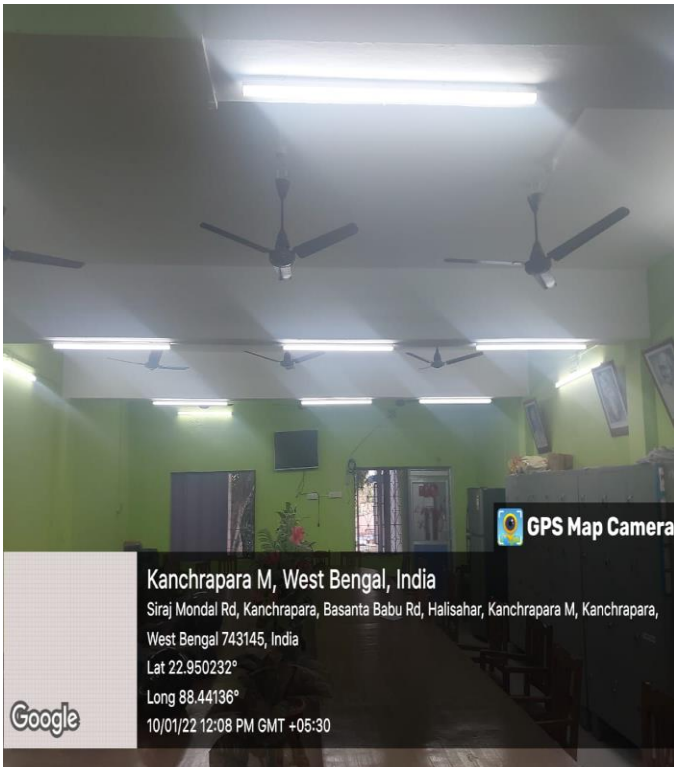
LED LIGHTS IN STAFFROOM
